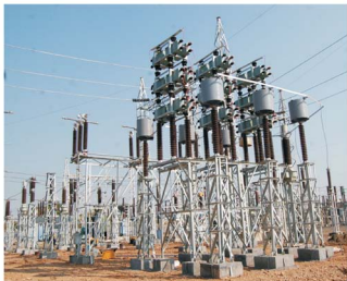
MSETCL 132 kV Capacitor Bank
